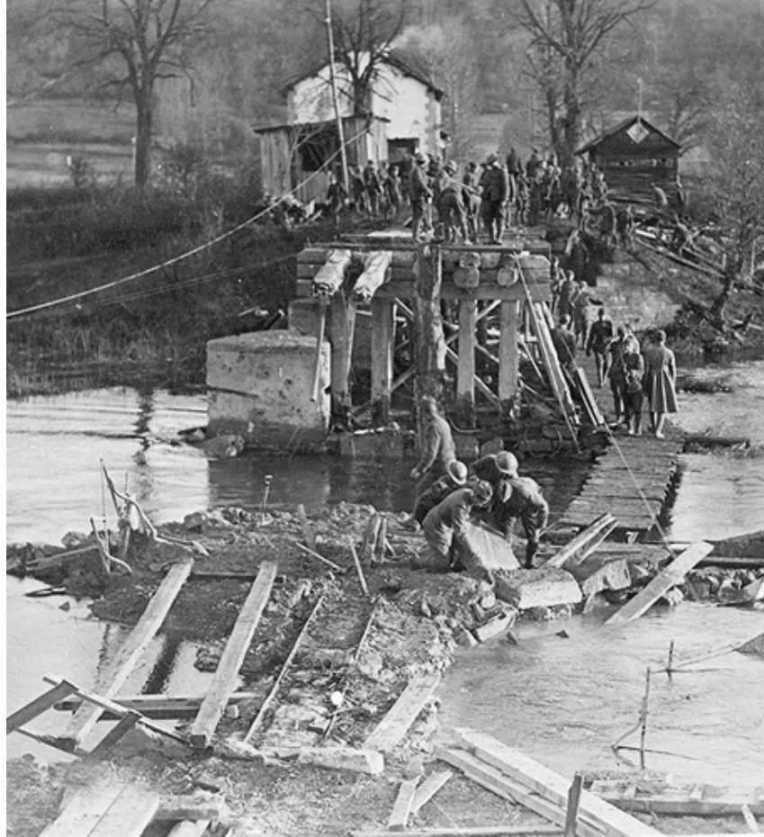
Engineers Building a Bridge Across the Meuse Near Pouilly After the Armistice
